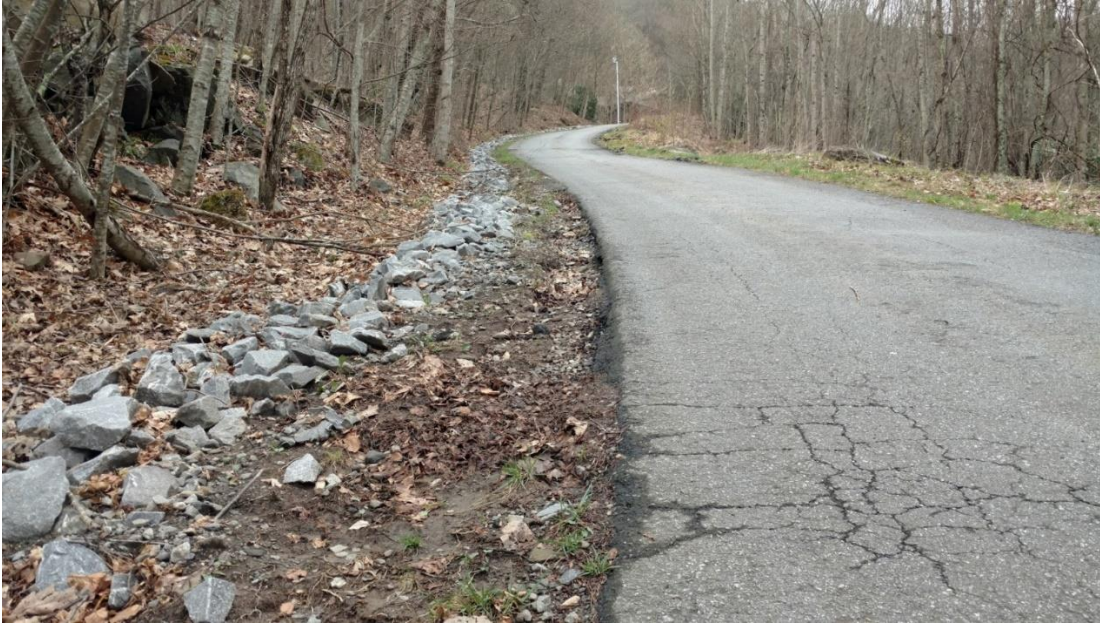
MLR near Carriers – Ditch repair required. Water diverted into road and eroding shoulder.
